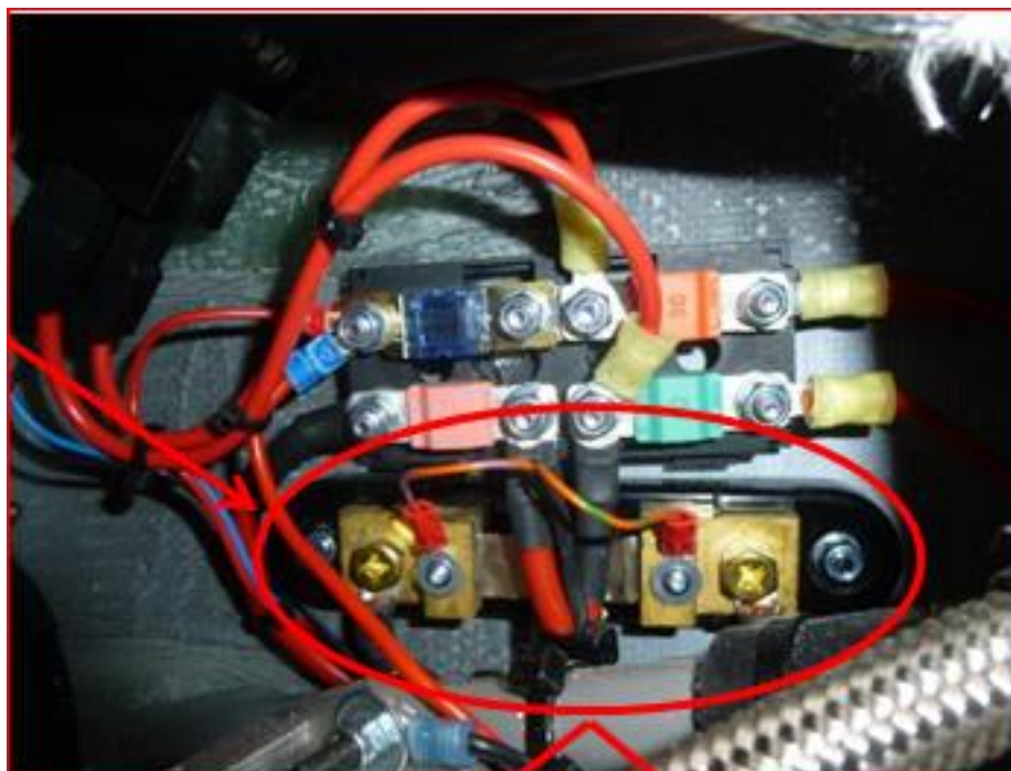
Fig 1: Shunt, old installation
