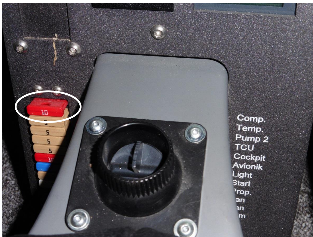
Fig. 1: 10A Fuse Compressor
